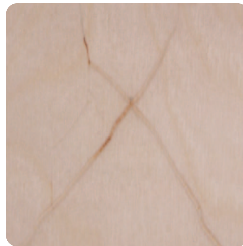
Traces of stringers
